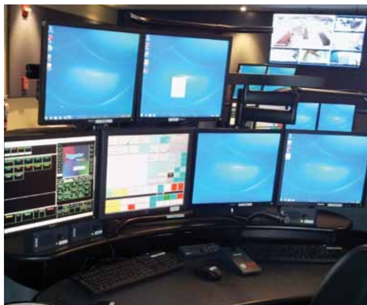
Multiple screens at an operator position in the SSRECC.
